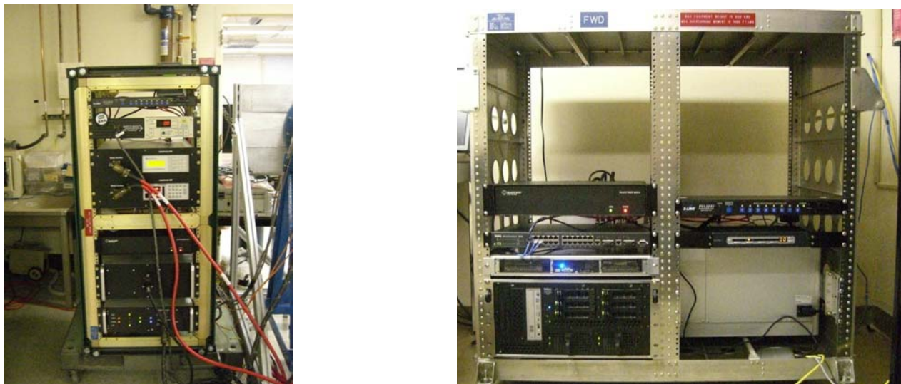
Figure 10: CW rack (left) and PI rack (right). The former contains instrument electronics and PI rack holds computers.
